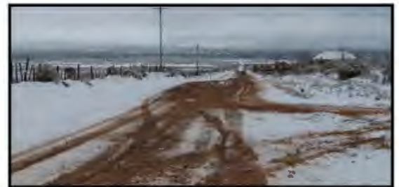
Cane Beds Road Post-Storm Condition
