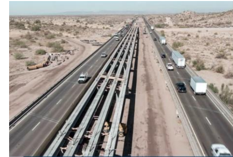
Construction of bridge girders for the Gila River on I-10 in Pinal County
